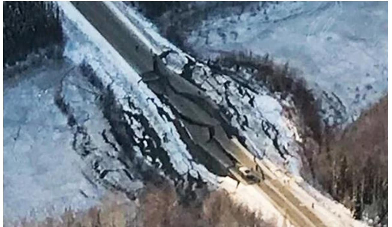
Magnitude 7.0 Earthquake Shakes Alaska, Damaging Roads, Buildings
